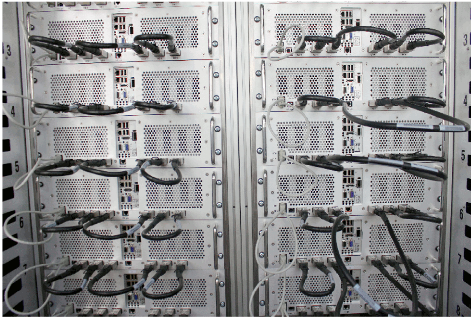
Fig. 4. Close-up view of the Janus II machine installed at BIFI (Zaragoza). The installation has 16 Janus II boxes (12 are visible in the picture). The cables supporting the data-links in the z direction are mounted in loop-back mode for test purposes.
